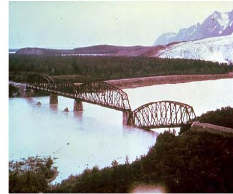
Failure of a bridge due to span losing support in the Prince William Sound, Alaska Earthquake
