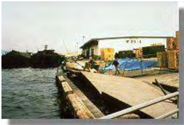
Retaining wall damage and lateral spreading, Kobe 1995
