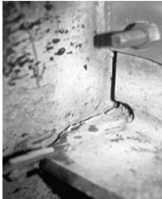
Failure in welded connections.
